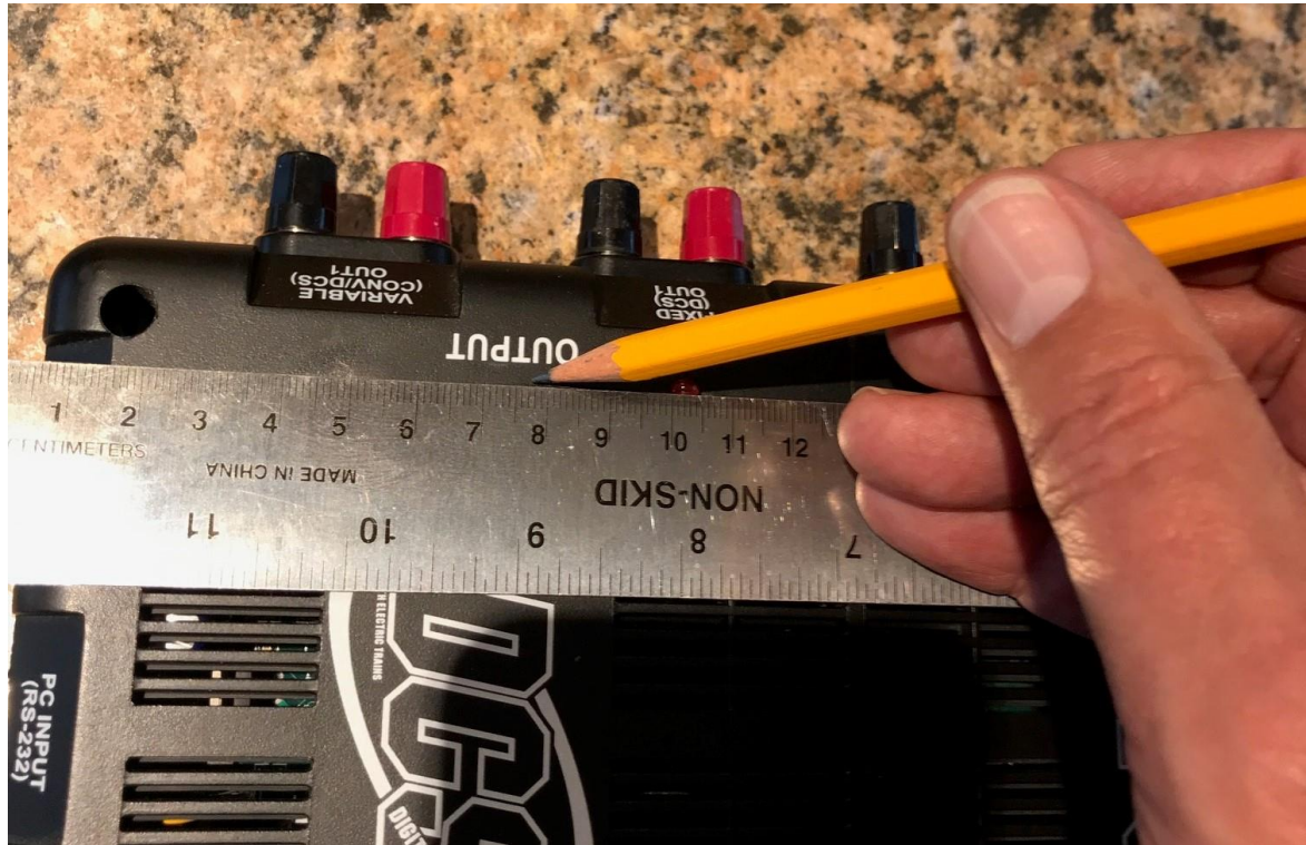
PIC 1; Draw a horizontal LED hole centerline 20mm away from the vents
