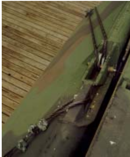
Figure 3. Close Up of the Top Lifting Eyes of the Bridge Bay Used for Tiedowns.
