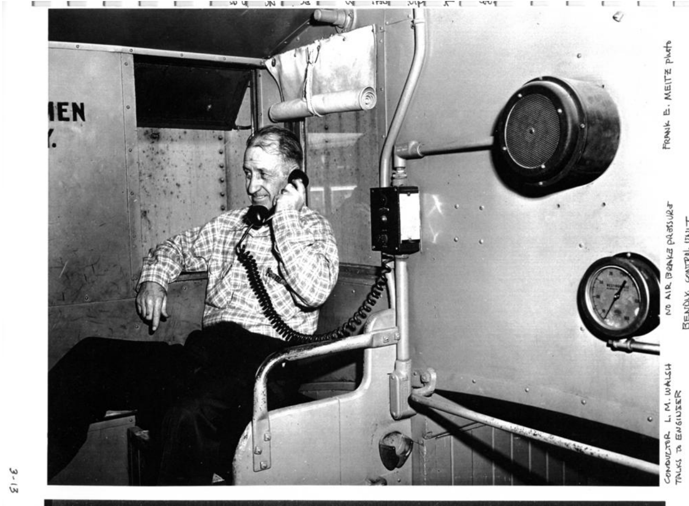
Typical view of cupola and installed radio equipment - sun shade for end windows
